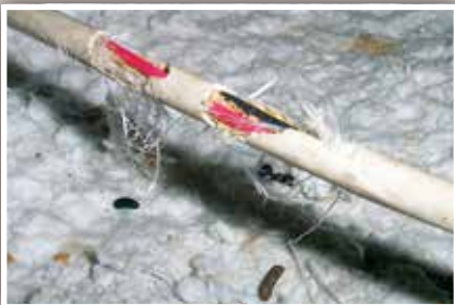
Gnawing on wires with droppings.*
