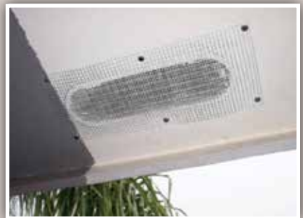
Soffit vent hole sealed with screen.*
